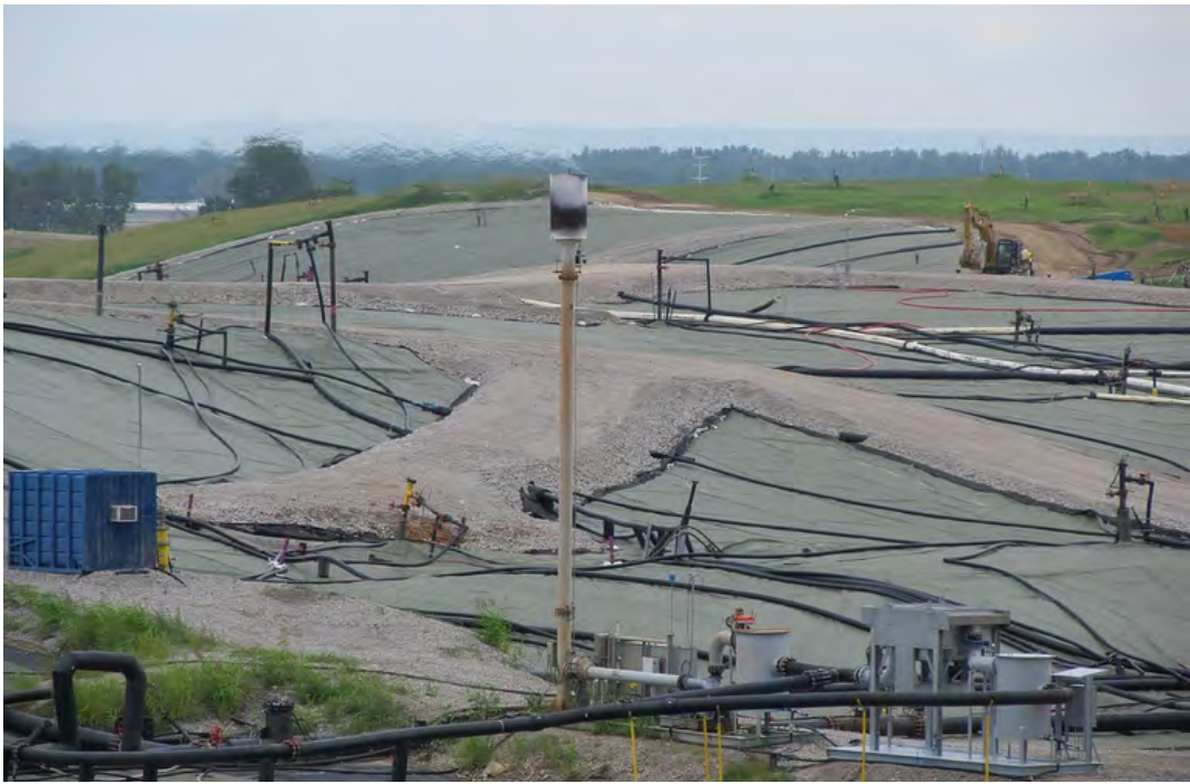
Westlake Landfill, where you can see the equipment used to extract gases from the landfill and burn it off
